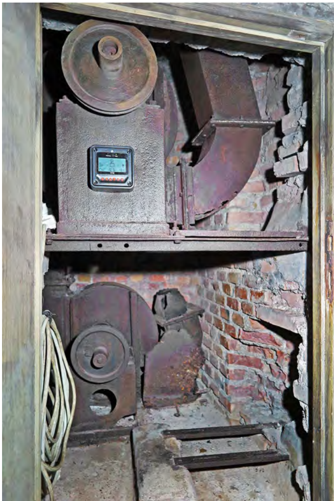
Ventilation equipment at the Villa Ada shelter. Batteries are now housed out of sight, but the status gauge is visible
